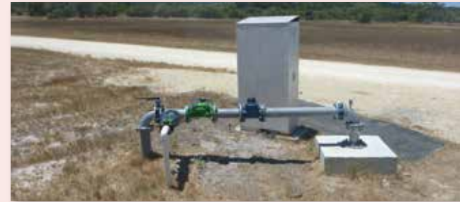
Water meter installed on galvanised headworks. Direction of flow is R to L.
