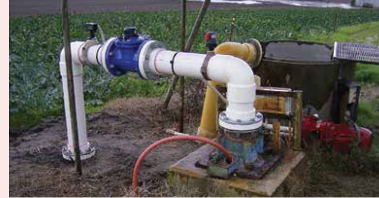
A correctly installed meter. It has no off-takes before the meter, and the required amount of pipe either side of the meter.
