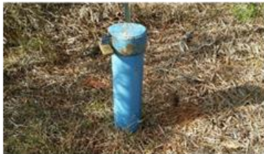
Painted steel headworks (without ID stickers)
