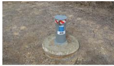
Painted steel headworks (with ID stickers)
