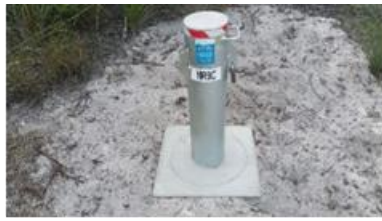
Galvanised steel headworks
