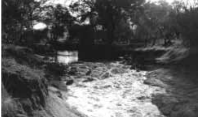
Figure 2. Riffle structure located 80m upstream of the Spencers Brook confluence with the Avon River in full flow during June 1998. The pool upstream extends for approximately 160m.
