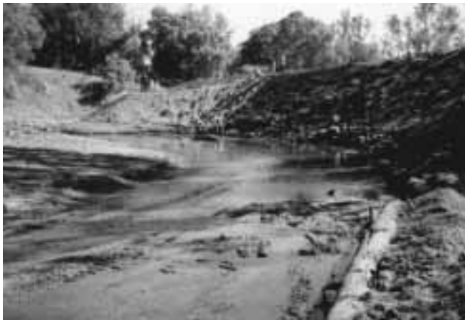
Figure 10. Works in progress on the Brunswick River. Large logs and boulders were placed along the base of the eroding bank (foreground) and the face battered and covered with matting (background).
