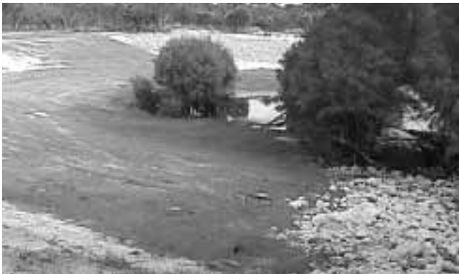
Figure 12. The channel was filled and battered in July 2000. Rock was placed to protect the entrance to the break-out channel.
